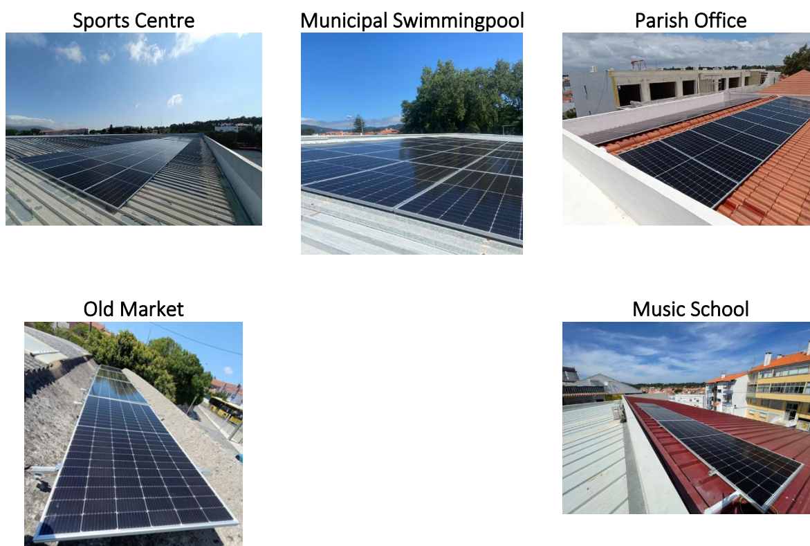
Figure 29 – PV systems in the 5 building's rooftops
