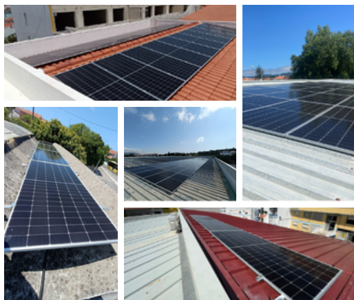
PV panels across the first five buildings in Alcabideche
